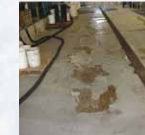
Failed epoxy flooring due to excessive water vapor transmission.
