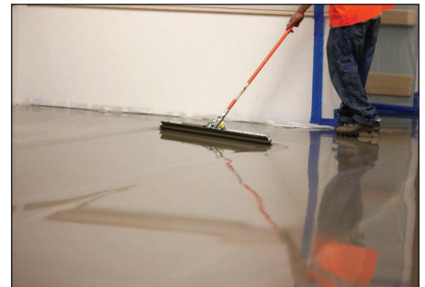
Using a spreader or gauge rake ensures even and uniform placement of the AQUAFIN LEVEL-Ultra.
