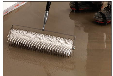
After placement a spiked roller is used to de-aerate the AQUAFIN LEVEL-Ultra, preventing pin-holing and surface dimpling.
