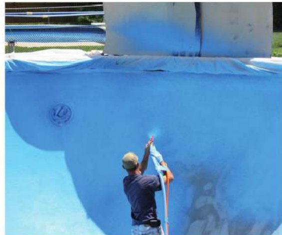
Spray equipment can be used to apply waterproof coatings on large surfaces.
